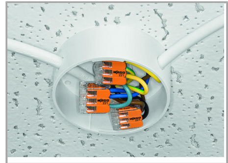
Lighting distribution in ceiling canopy
