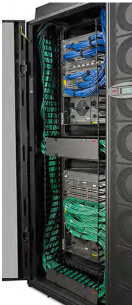
(2) Cisco Catalyst 6509 – AR3140 Enclosure and AR7715 Side Airflow Duct Kits
