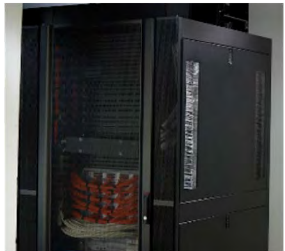
Installed on AR3340 enclosure
