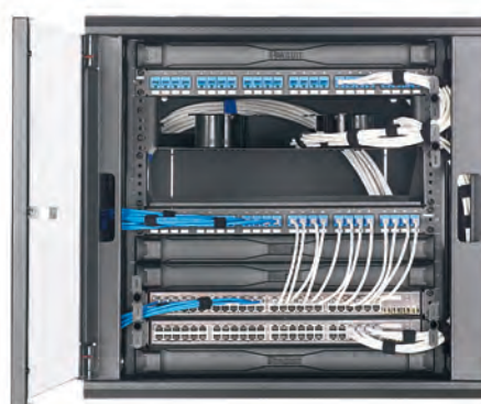
Figure 1: Application of a horizontal slack manager and bend radius posts installed in a wall mount cabinet
