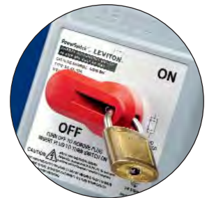
Handle with padlock installed
