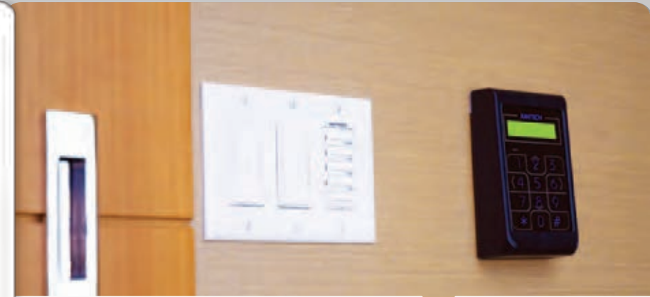
“Stand-alone proximity access control system”
