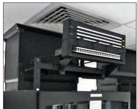
View of PatchRack installed on CPI Cable Runway above CPI Cabinet.
