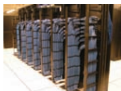
ICKC shown installed
