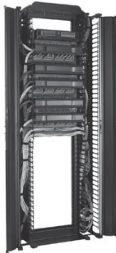
Vertical and horizontal cable manager system installed on a 2-post rack. Vertical and horizontal cable managers work together to make an orderly installation.
