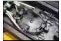
Installed Fiber Organizer for Ribbon
