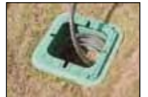
Slack Cable Storage in Small Base
