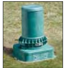
Installed 17" (453 mm) GLC with Grounding Spacer
