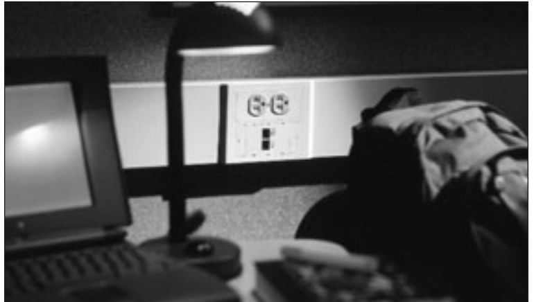
4000 Series Raceway in a typical dorm room application.
