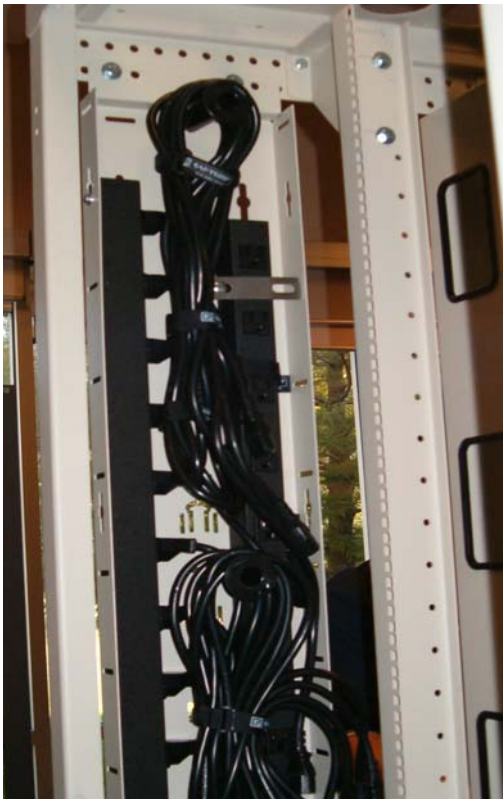
Fig. 5.2.1 Bundled power cables
